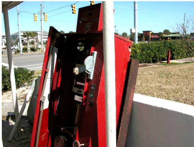
Old fire pump controller.
