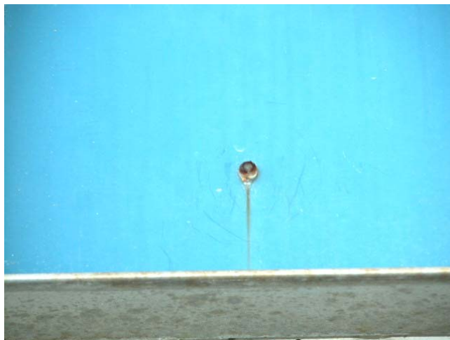
Corrosion of fastener that holds metal panel in-place.
