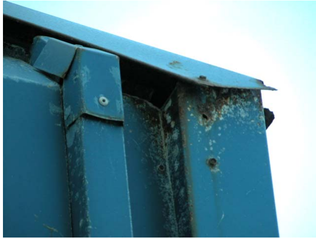
Corrosion damage at roof corner.
