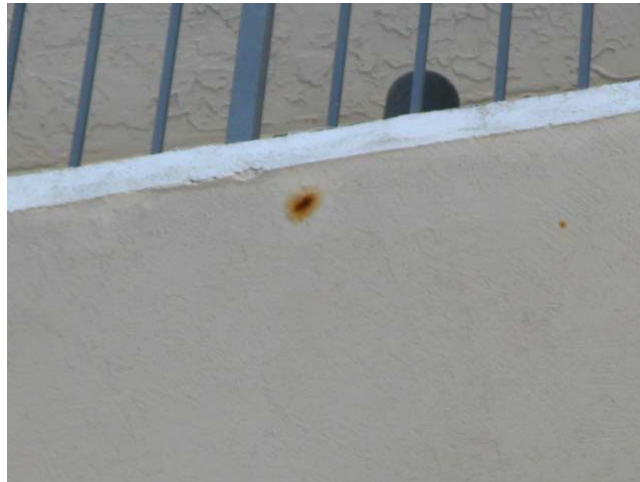
Rust spot forming on the concrete of a balcony.
